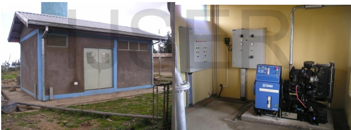
Figure 3. 4 View of the Pumping Station at R2
