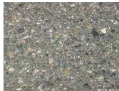
Figure 1: Road surface showing polished aggregates
