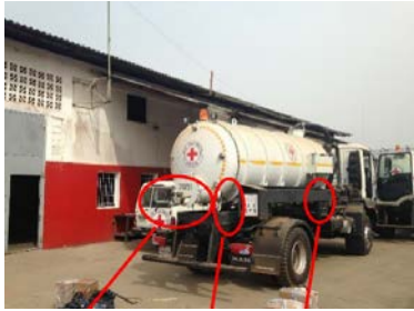
Figure 4. Sewer truck containing inlets/outlets connections, pump mode and control panel used for transporting sewage to the Treatment plant
