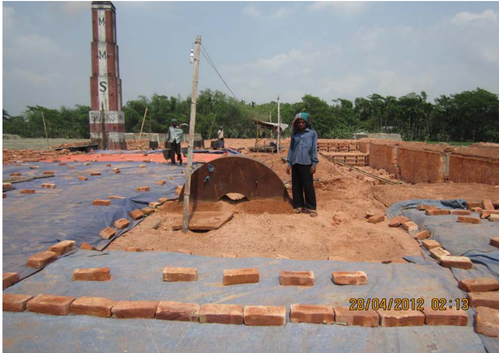
Fig-3.1: Zigzag chimney (Firing condition)
