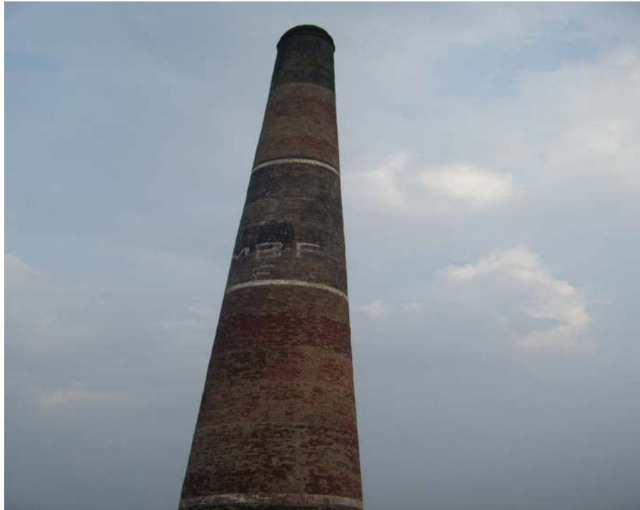
Fig-3.3: Fixed chimney
