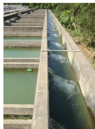
Fig 3.19: Clean water is collected from the upper part of the clarifier
