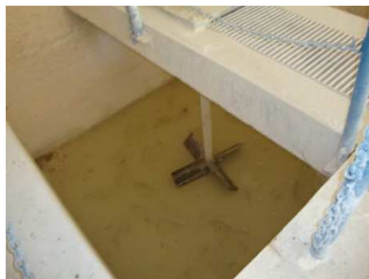
Fig 3.25 : Lime mixing tank
