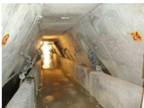
Fig 3.22: Wastewater drain below clarifier
