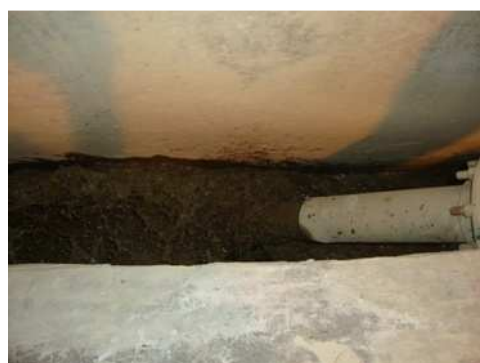
Fig 3.23: Waster discharging from clarifier
