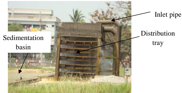
Fig 3.27: Aeration tower and Sedimentation Basin
