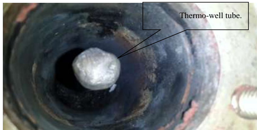
Figure 14: thermo-well inside heater cylinder.
