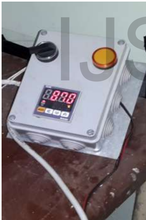
a) Temperature controller
