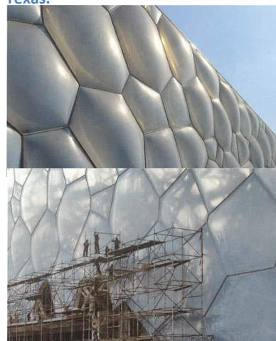
Figure 3.24: The pattern of the building shell of the Watercube, the National Swimming Centre for the 2008 Olympic Games in Beijing, China, resembles oversized buckyballs, but has otherwise nothing in common with nanotechnology.
