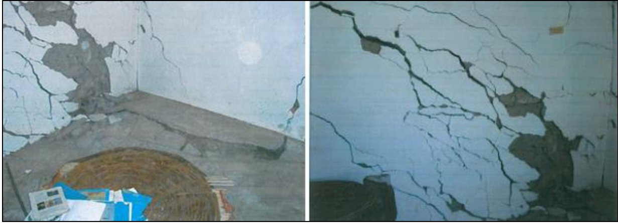
Figure 3.7: House damaged due to failure of slope at terraces (Hussain & Awan, 2009)
