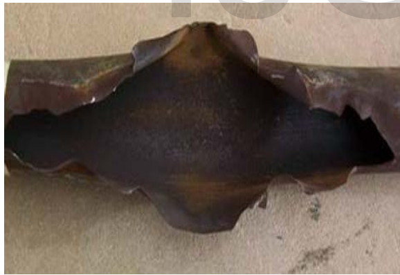
Figure 9. Photograph showing economizer tube in as received condition
