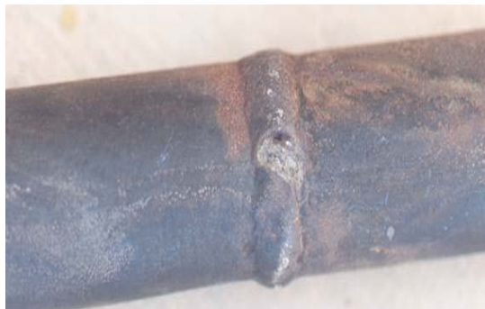
Figure 2. Photograph of economizer tube showing frontal view (Side A)
