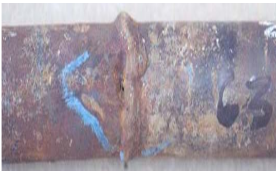
Figure 13. Photograph of the economizer tube A in as received condition showing (closer view)
