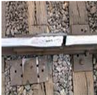
(Fig7.1Detection of cracks)
